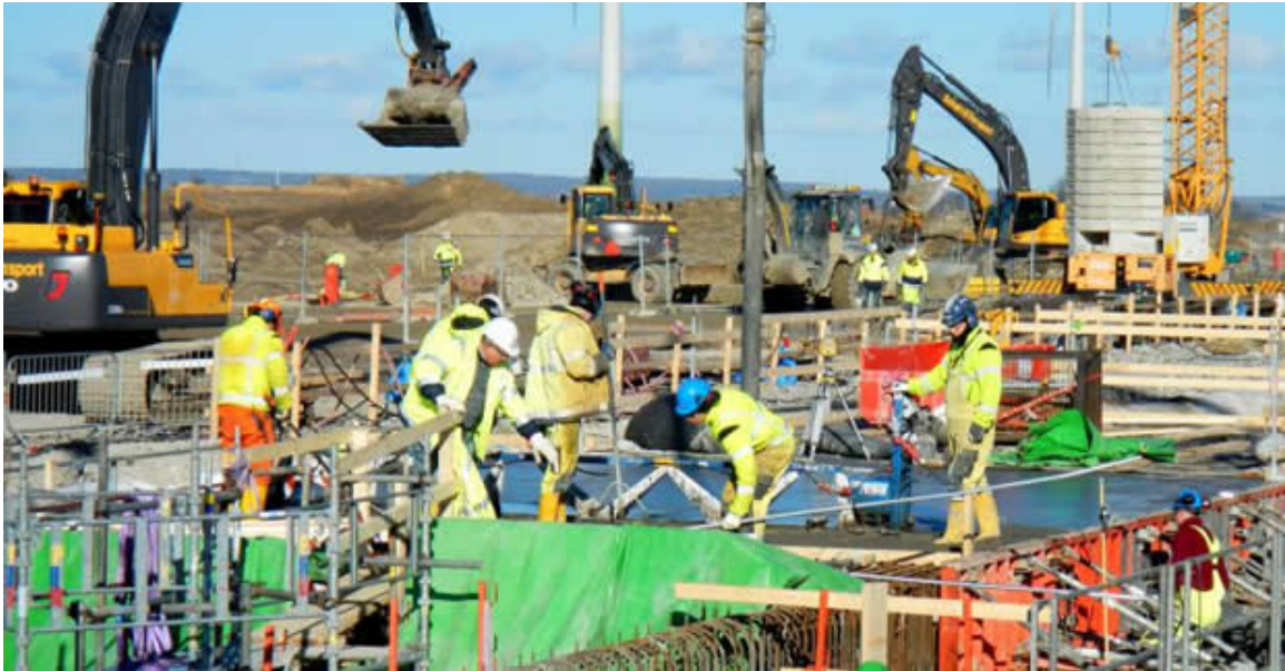
Workers managing the concrete pour for casting a section of the vault, or roof, of the ESS Accelerator tunnel.
